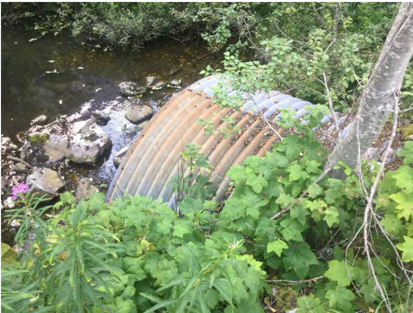
Typical Light Corrosion on Top of Inlet & Outlet
